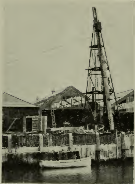
FIG. 12.—QUAY WALL AT LOWESTOFT: FRONT SHEET WALL AND YOKE PILES BEING DRIVEN.
